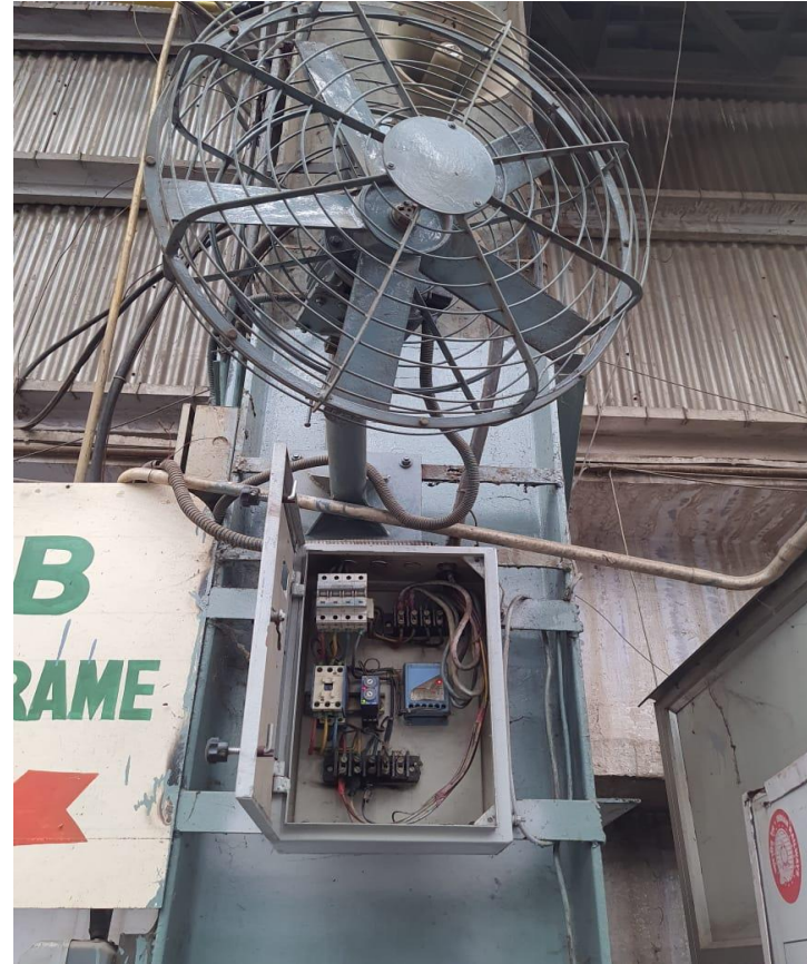
TIMERS PROVIDED IN MANCOOLERS CIRCUITS
